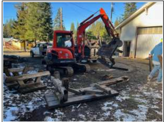
Forest Service employee Blair Anderson delivers the first load of picnic tables to our Natural Resource Center for Wood Shop refurbishing.
