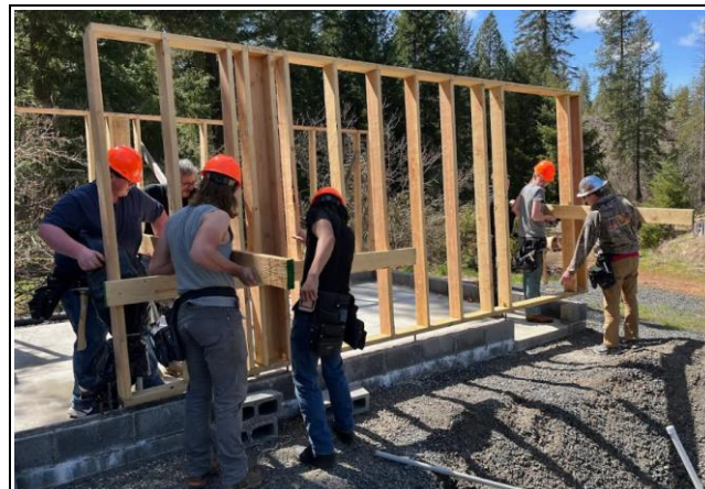
Another section of wall framing is set in place and secured. And it fits with great accuracy!
